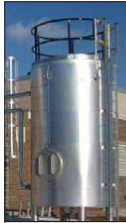
WAUSAU WATER WORKS, WI
